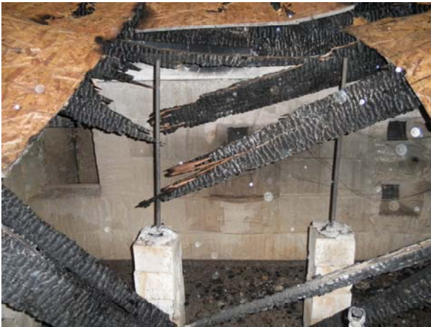
Figure 83. Joist rupture in center span
