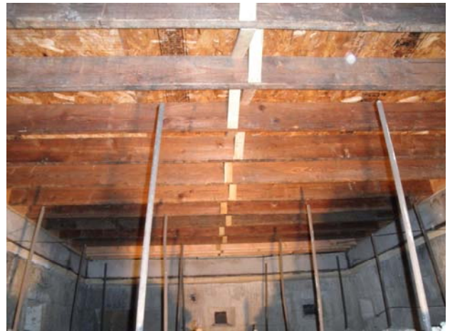
Figure 86. Pre-test exposed side
