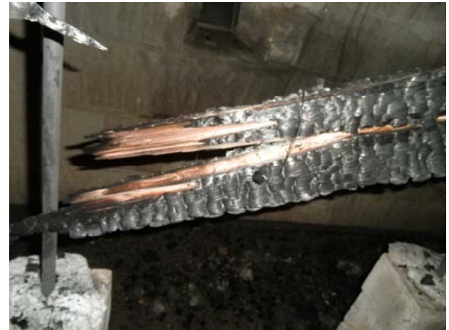
Figure 84. Close-up of joist rupture
