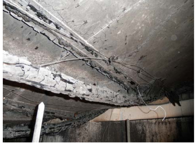
Figure 72. Close-up of some remaining web
