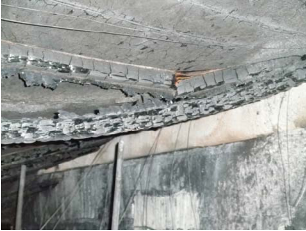
Figure 71. Joist with web burn through
