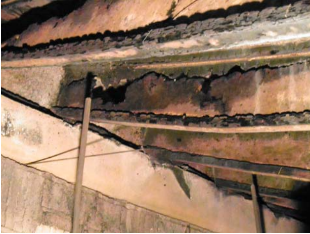
Figure 47. Joist with web burn through
