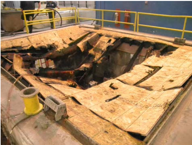
Figure 93. Unexposed side after collapse
