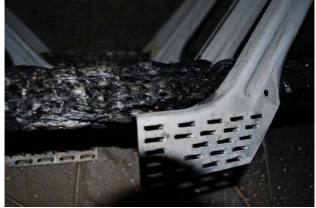
Figure 36. Close-up of char depth
