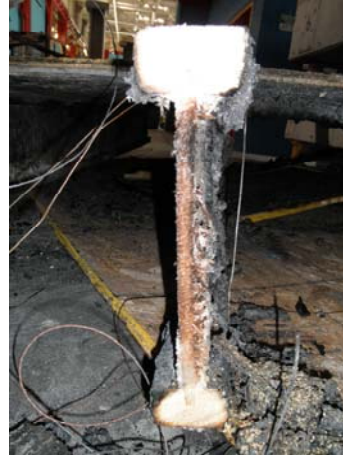
Figure 48. Close-up of remaining web
