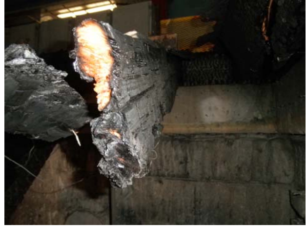
Figure 96. Close-up of joist rupture
