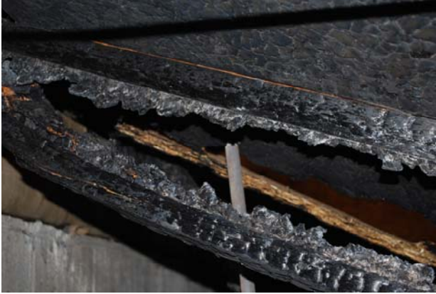
Figure 59. Joist with web burn through
