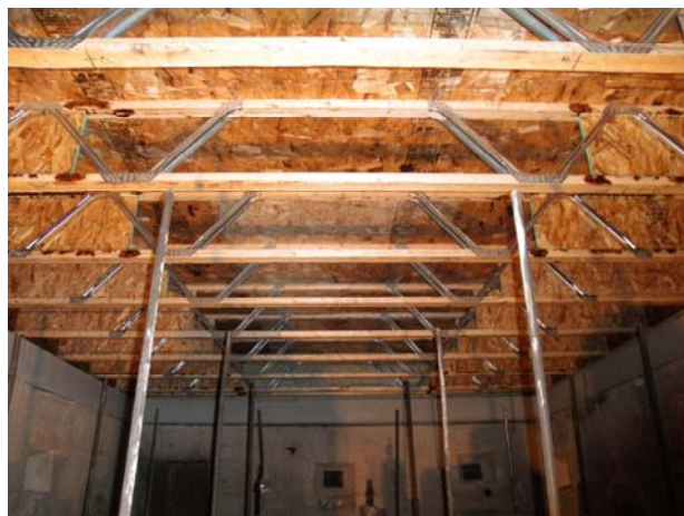
Figure 26. Pre-test exposed side
