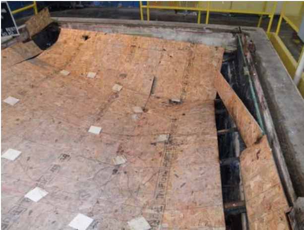
Figure 69. Unexposed side after collapse
