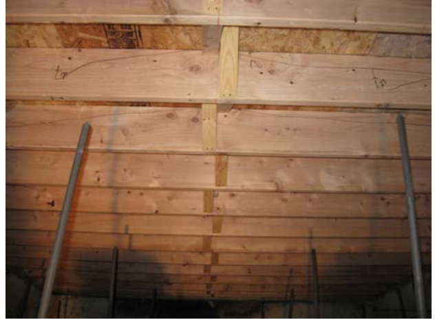
Figure 74. Pre-test exposed side
