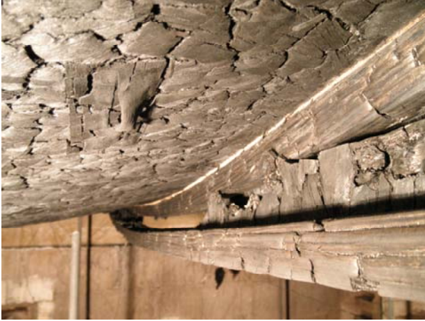
Figure 23. Joist with web burned away
