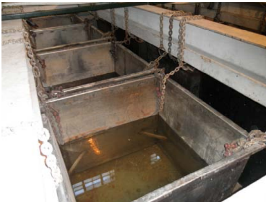
Figure 10 - Steel Tanks Filled with Water
