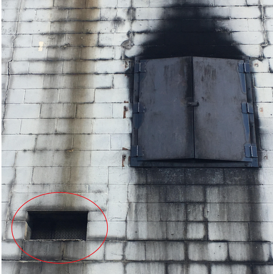
Figure 3.17: Example of scupper along base of wall on second floor of concrete live fire training building
